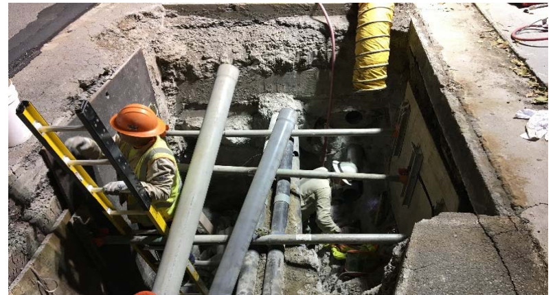
DWP Power Duct Bank and Conduits
