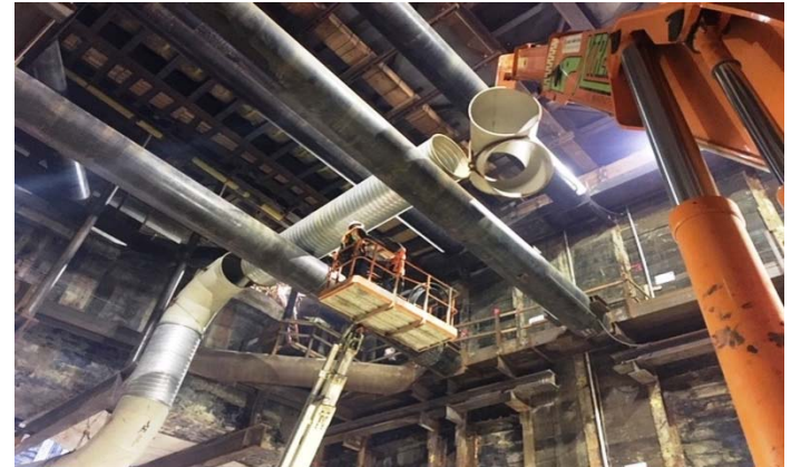
Reconfiguration of Ventilation at the Western Shaft
