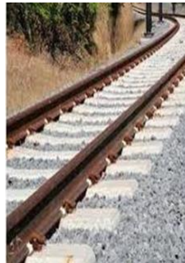
Figure 7: Concrete sleepers prevent deformation in rail
