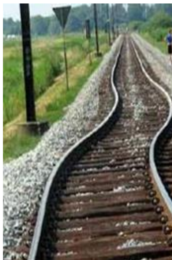
Figure 6: Sun kinks occur with wooden ties
