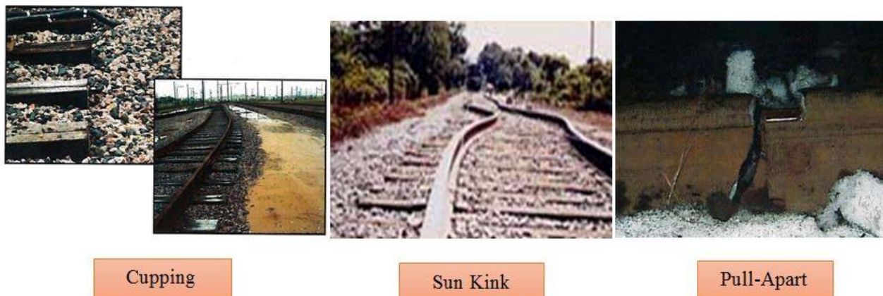
Figure 12: Photos of rail "cupping," "sun kink," and "pull-apart"
