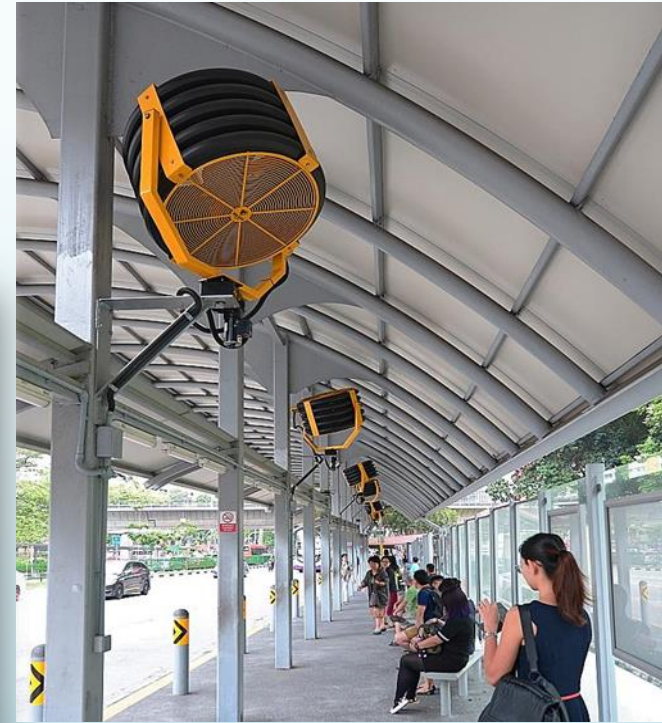
(10) Electric fans at bus stop
