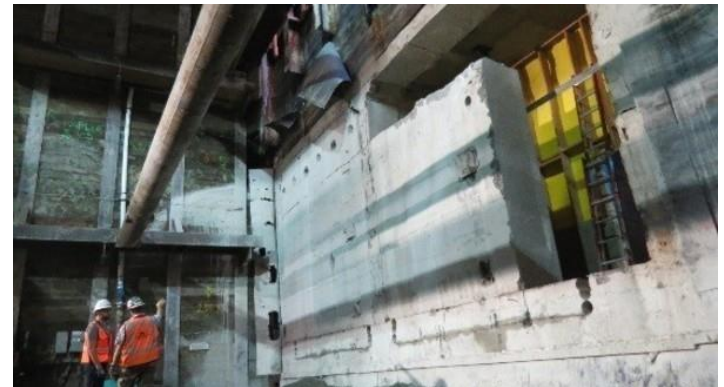
Break through knock-out panel at 7 th /Metro Center Station
