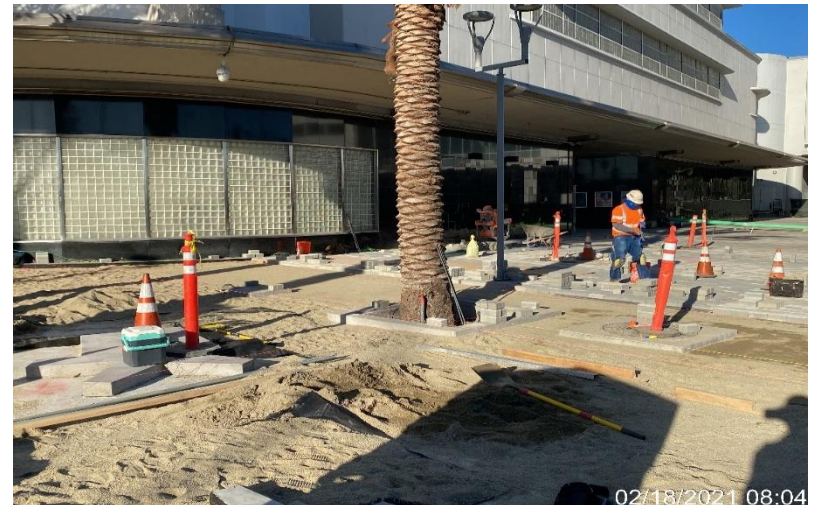
MLK STATION – Continue brick paver installation at the north end area of the plaza.
