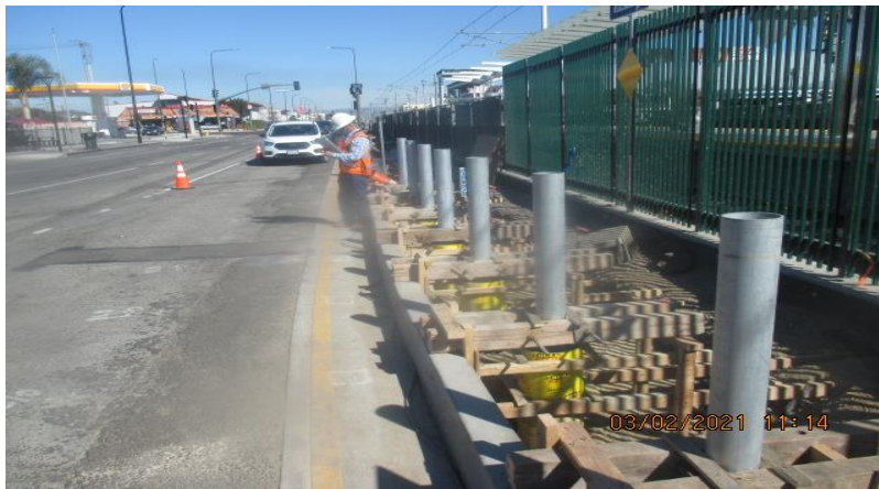
HYDE PARK STATION – Building formwork and installing bollards along the southbound median of the station.
