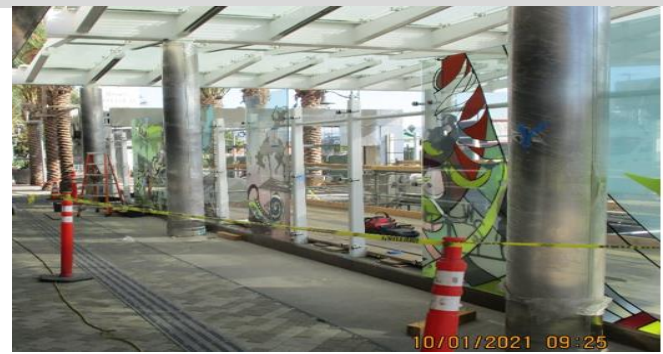
MLK Station – Art glass panel installation around the perimeter of the main entrance canopy at the plaza.
