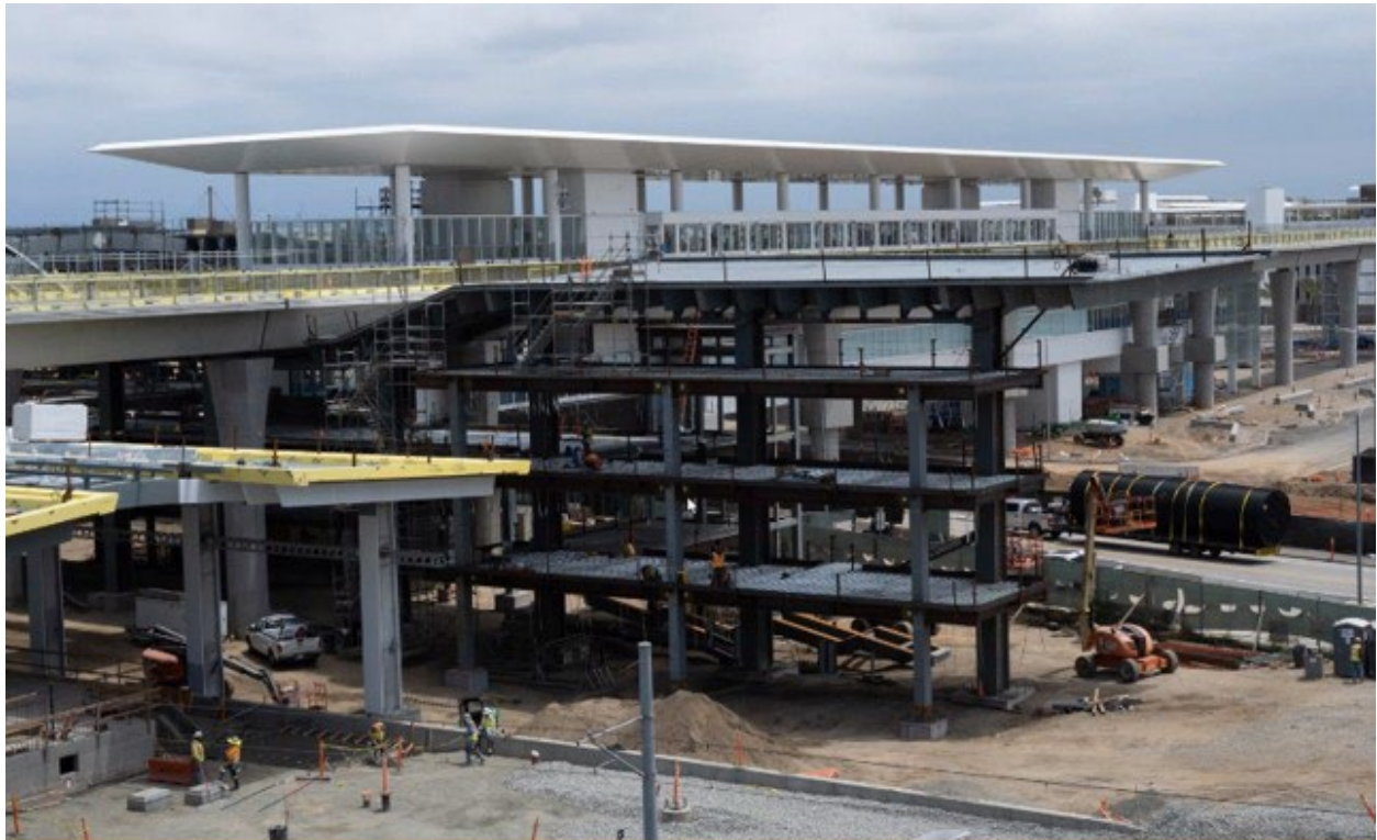
Airport Metro Connector and Los Angeles Airport Automated People Mover construction site
