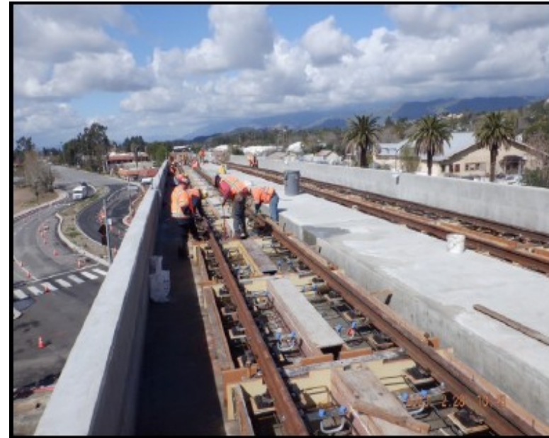
Bonita / Cataract – Structure Track Direct fixation
