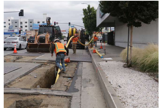
Installation of a 4" gas main by SCG on Van Nuys Blvd, just south of Saticoy.
