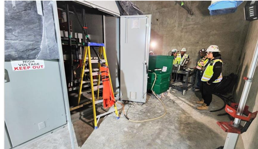
Wilshire/Fairfax High Potential Testing of High Voltage Cable
