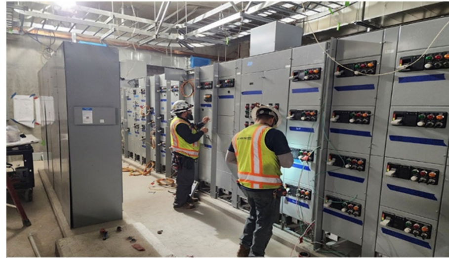
Wilshire/Fairfax Testing Motor Control Center
