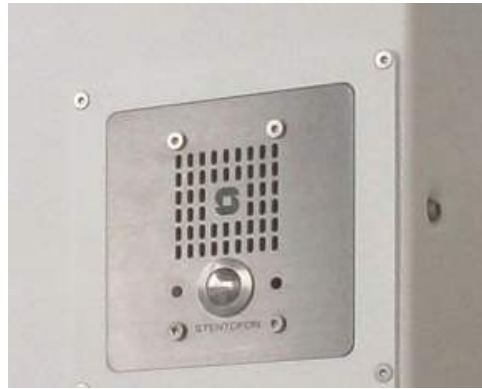
Image 34 – In-Cabins Call-Button and Intercom
