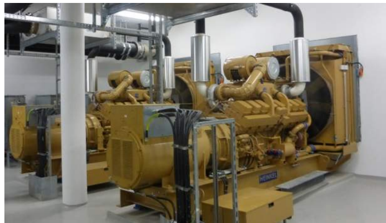
Image 43 – Backup Power Generators
