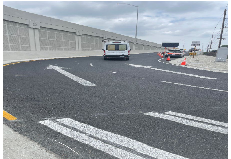
NB 405 South of Van Ness Blvd (SW #760) with completed retaining concrete barrier at 186 th Street
