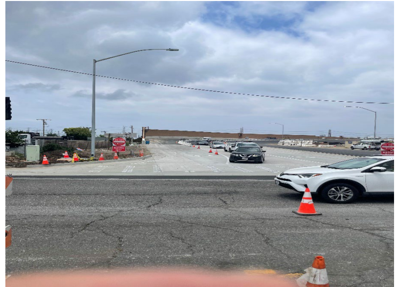
NB Crenshaw Blvd to SB 405 on ramp (RW#803) completed concrete barrier slab (Looking North)
