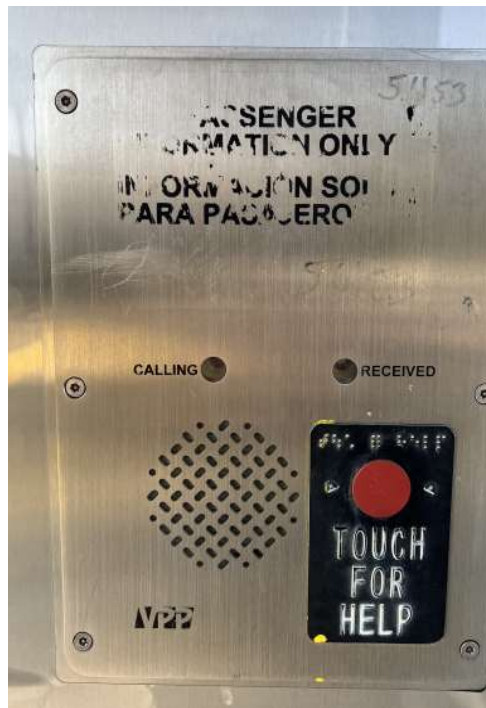
Picture 3: E Line – Expo/Crenshaw Extension 56153 – Faded Number
