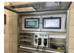
Wilshire/La Brea Station: Testing Emergency Management Panel
