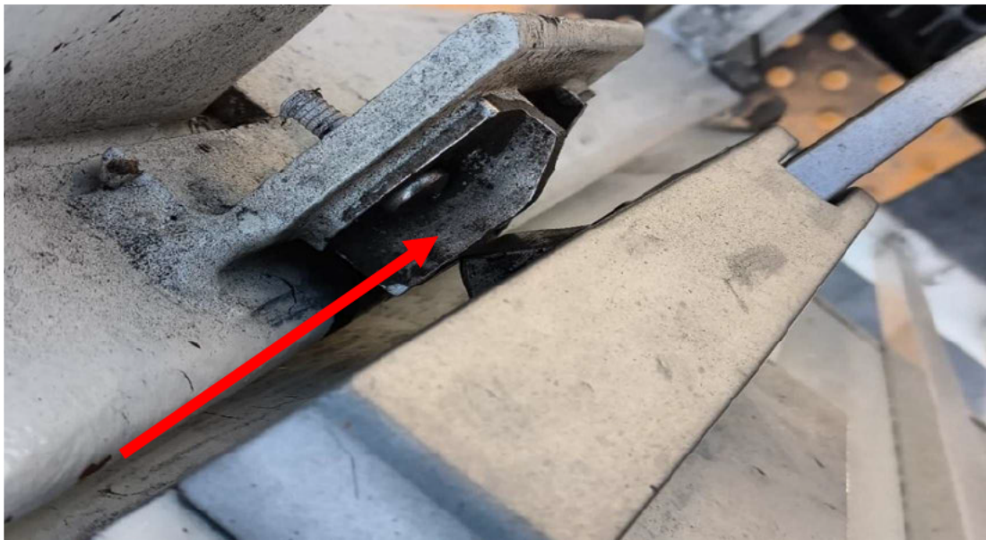
Leimert Park Station: 2024K-001 July 29, 2025 - Broken Latch
