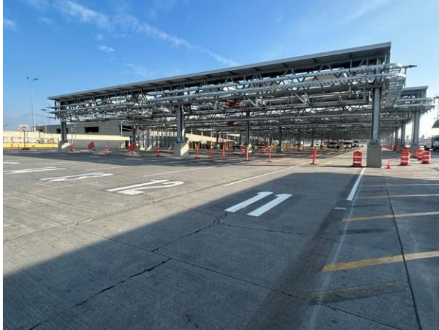
Division 9 Charging Station
