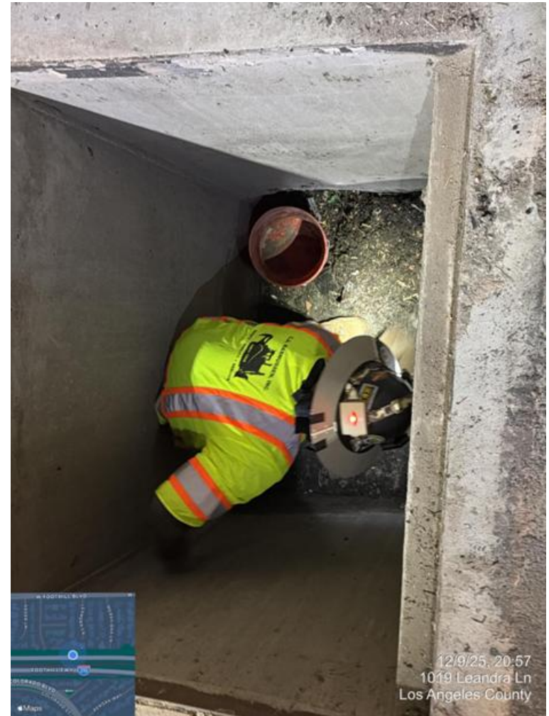
Irrigation pullbox per Punchlist (Arcadia)
