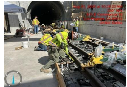
East Portal Tracks switch rods
