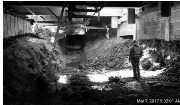
Utility hanging under 2 nd Street decking
