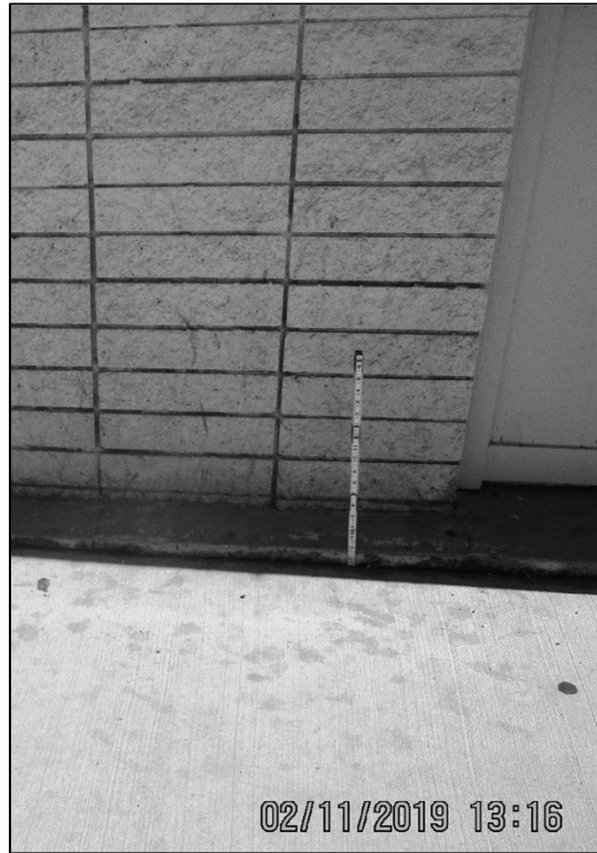
Back-of-walk lippage w/private property (Crenshaw NB 57 th St )
