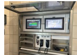
Wilshire/La Brea Station: Testing Emergency Management Panel
