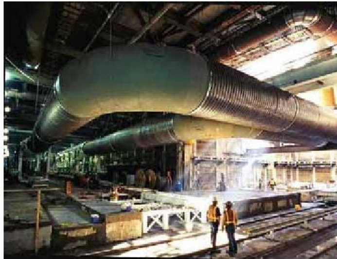
Figure 4-19: Underground Ventilation Ducts
