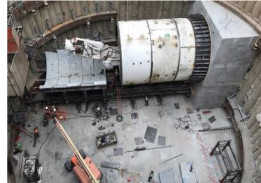
Installation of Temporary Invert Segments on Gantry Cradle at Base of Excavated Tail Track Exit Shaft
