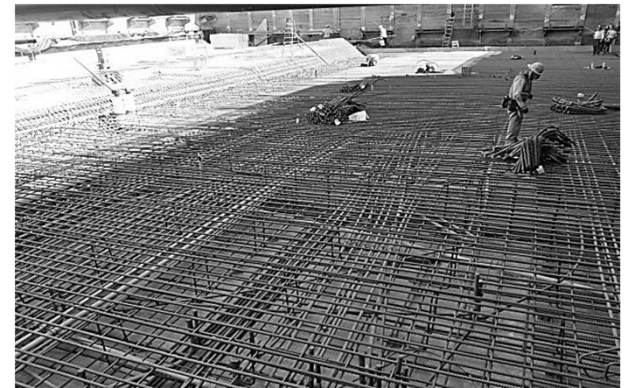
Installation of top mat of rebar and conduits for station invert at 1st/Central
