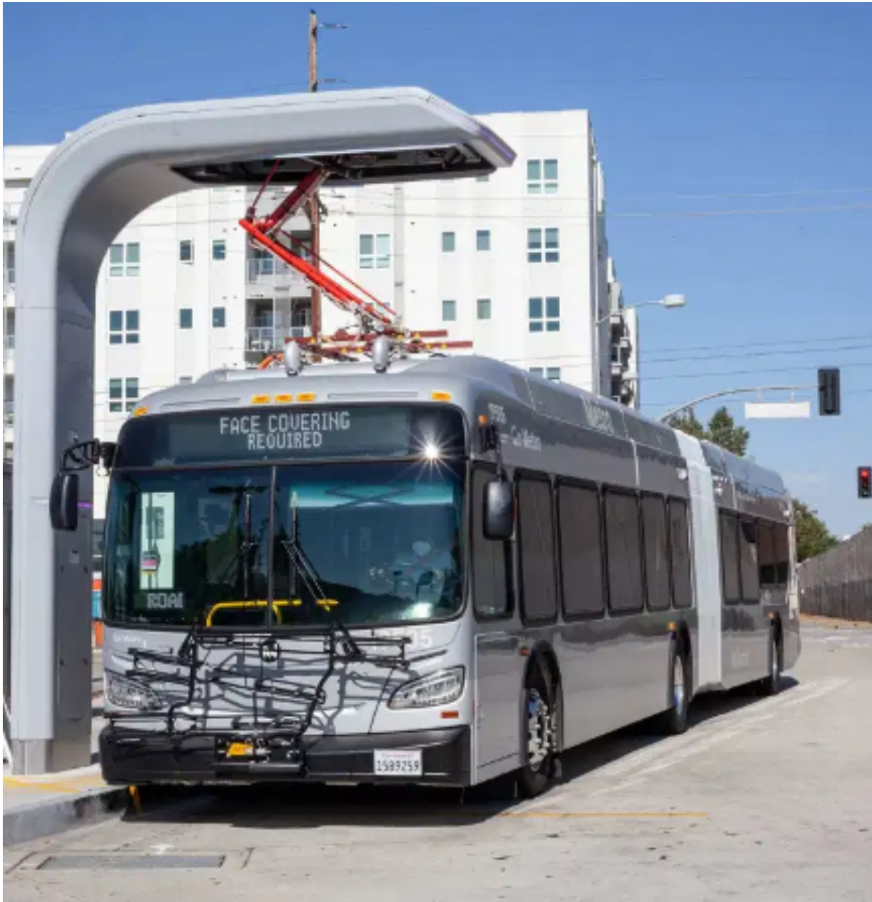
Figure 3-4. North Hollywood Station On-Route Charger
