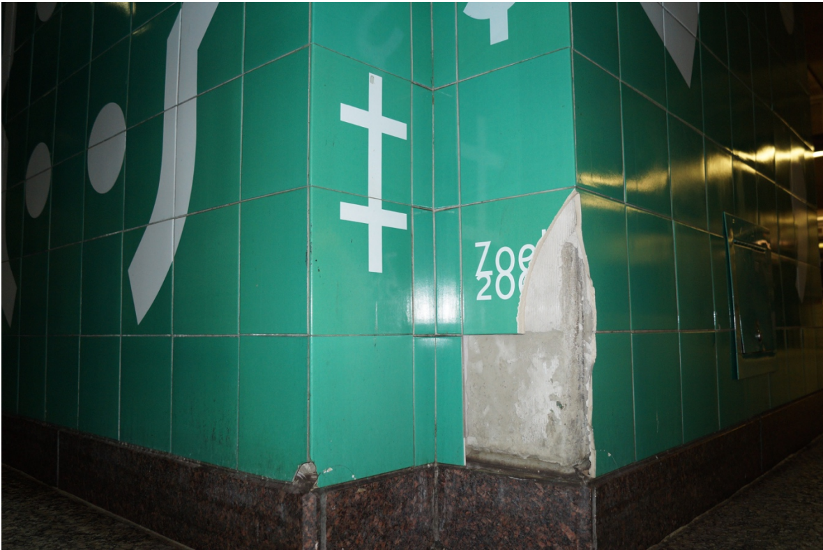
Metro Red Line – Damaged artwork tile requires specialized repairs
