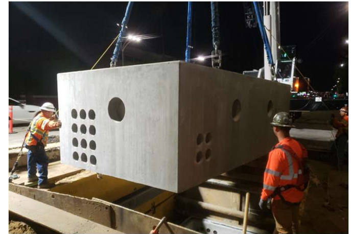
Installation of 1 of 4 vaults by on Van Nuys Blvd, between Vanowen and Vose.
