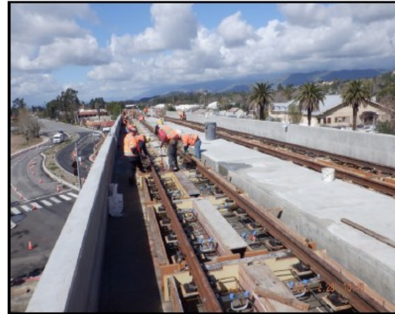
Bonita / Cataract – Structure Track Direct fixation
