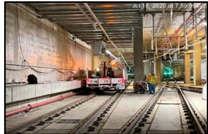
Continue installing supports and fixture for crossover lighting at the invert level of Expo/Crenshaw Station.
