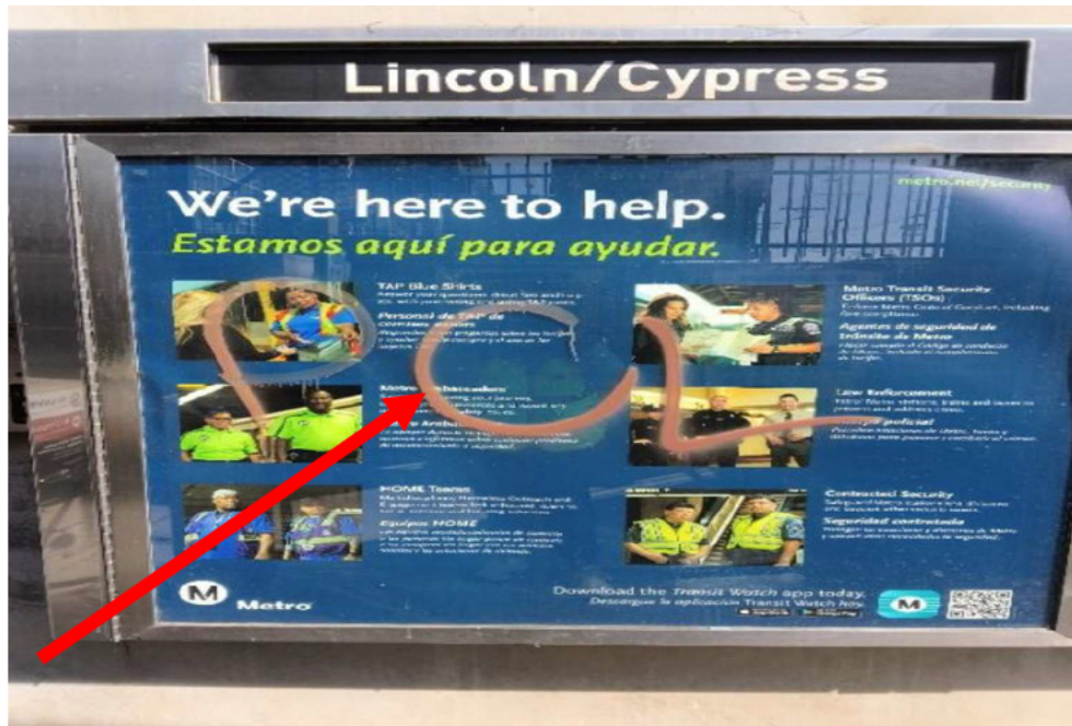
Lincoln/Cypress Station: 2024A-004 July 30, 2025 - Graffiti
