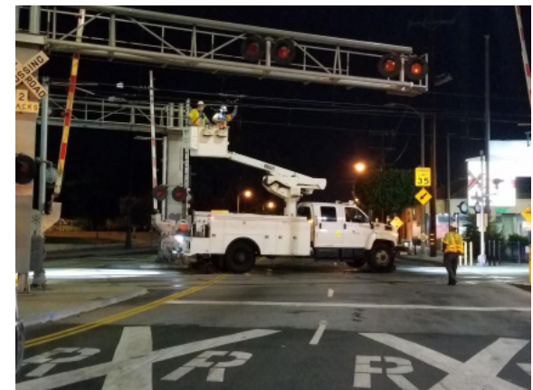
Traction Power Staff On-Site
