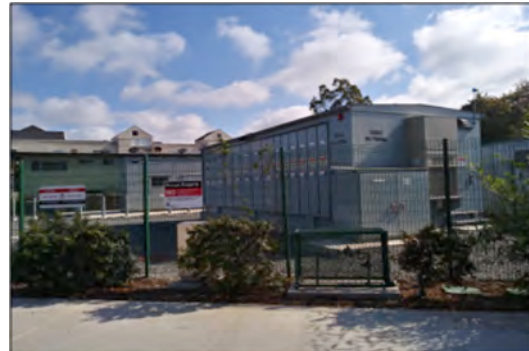
Photo ES-7: Typical TPSS for LRT
