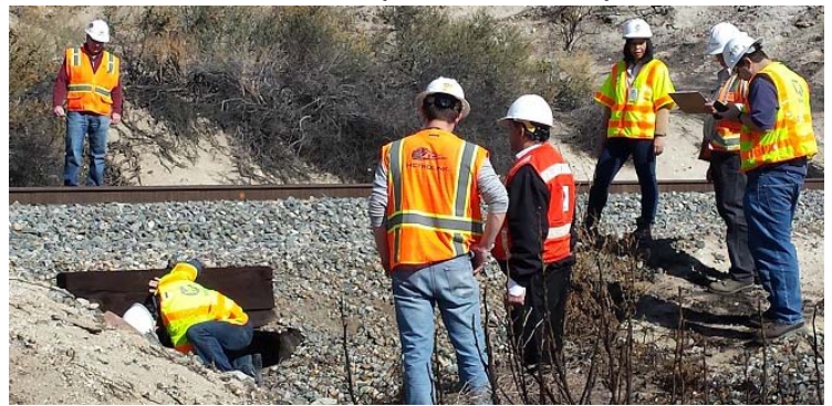
Picture 2: SCRRRA Staff and MTA Staff Inspecting a Wood Box Culvert on the Valley Subdivision
